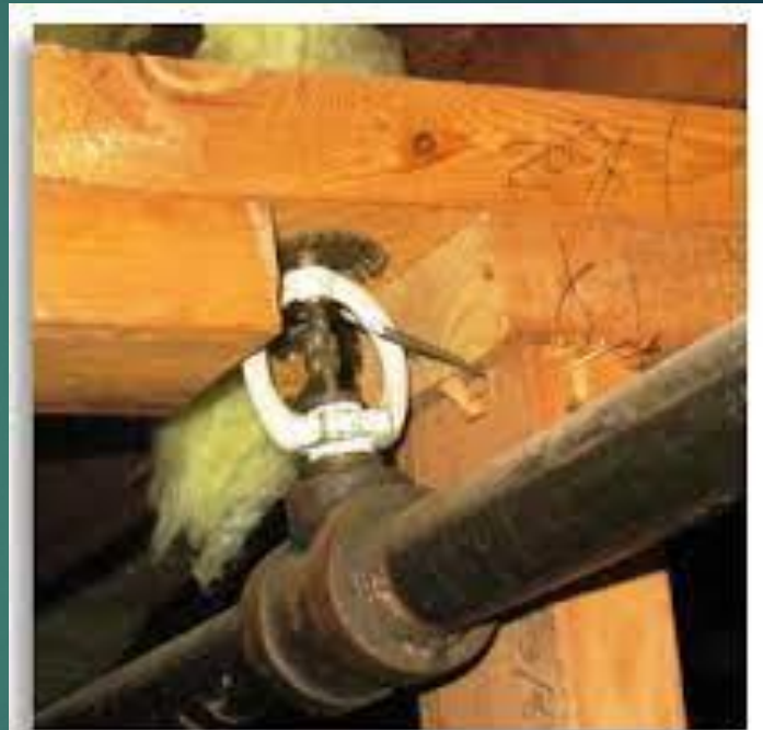
This upright sprinkler should be oriented with its arms parallel to the sprinkler pipe. Photo courtesy of Byron Blake.
