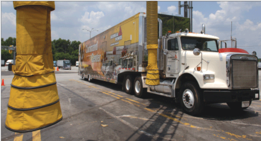
Figure 16. Electrified Truck Parking Space Equipment Photo courtesy of Georgia Power
